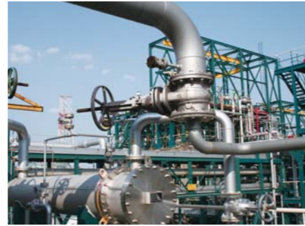
Gas recovery unit
